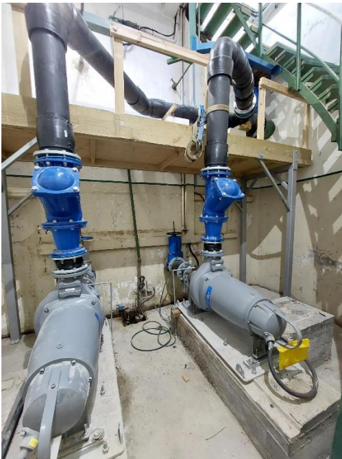
Figure 1-5: Fitzherbert Pump Station.
